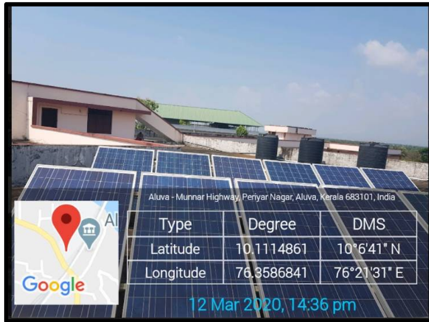
Fig. 6 Solar power Unit
